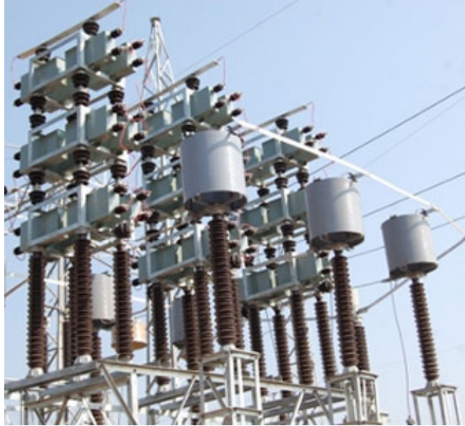
Figure 2.10. Shunt Capacitors. [Energie Capacitors]
