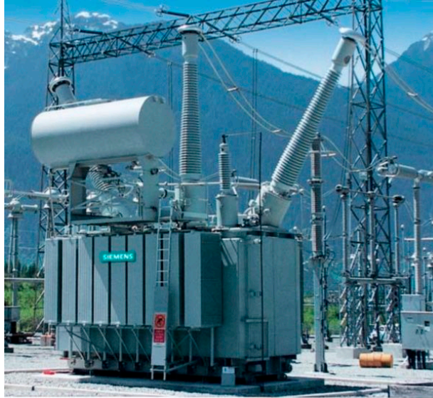
Figure 2.11. Siemens Shunt Reactor [13].
